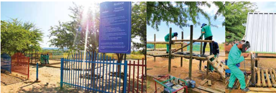
Community treasure: The Kornalyn playground in Khomasdal is open to the public again after repair work of over N$15 000 to damaged infrastructure was recently completed.
